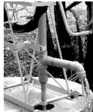
Size difference between riser pipe and upper pipe
