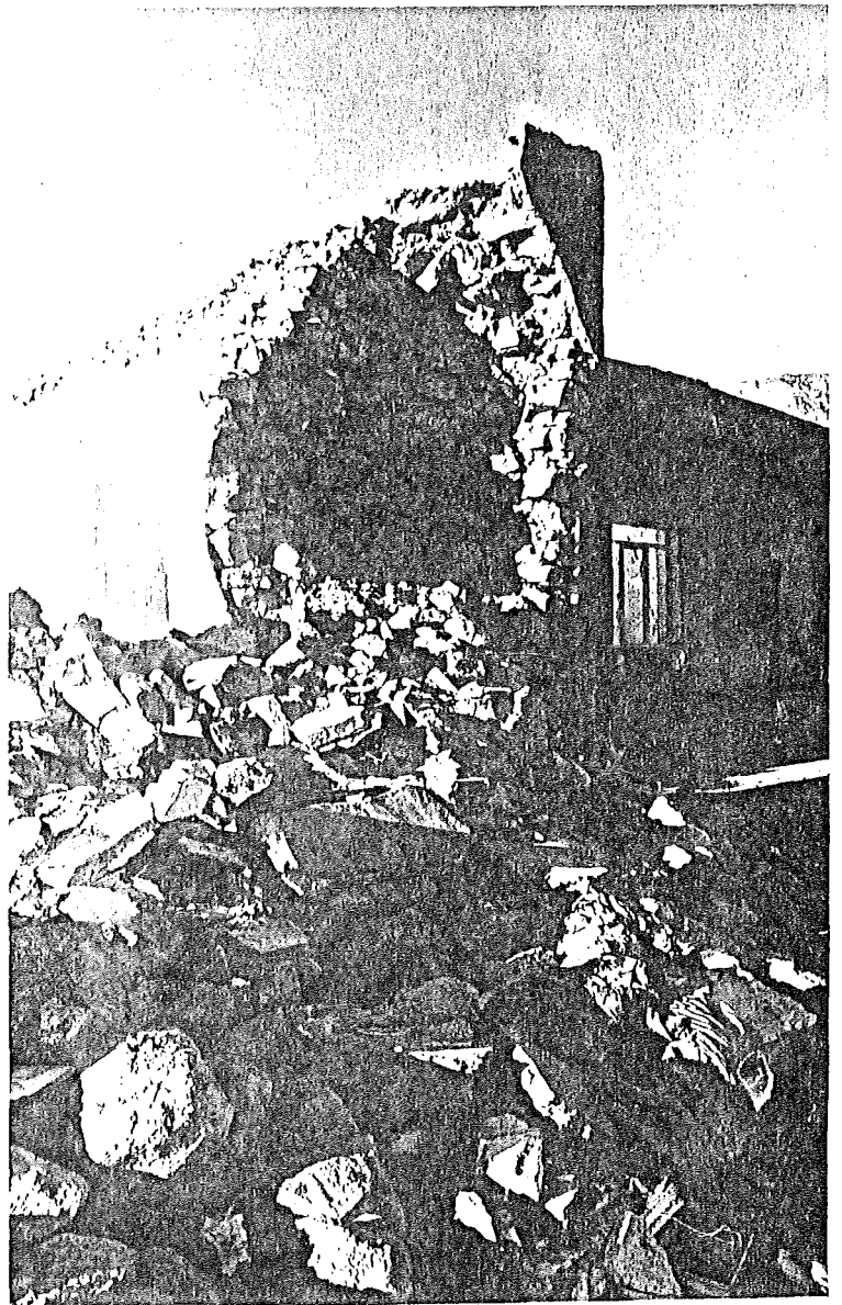
Sar Bagh: Corner failure due to stress concentration.
