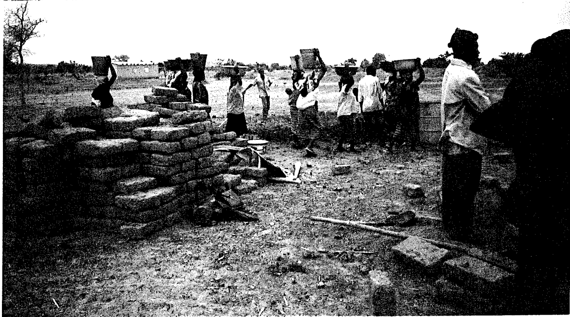
Photos 11 and 12: Village youth organisations in Burkina Faso undertake to provide the correct quantity of bricks, and on site earth, water and labour; only the skilled "woodless construction" building input is project-provided at this early "demonstration" stage.
