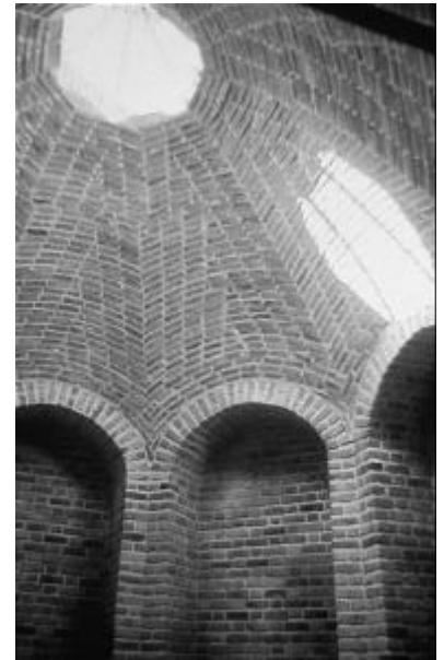
Fig. 4 The roof of the Niazabad public bath: in the '70s Development Workshop promoted the use of traditional Iranian vault and dome roofing in a series of public buildings in western Iran.
