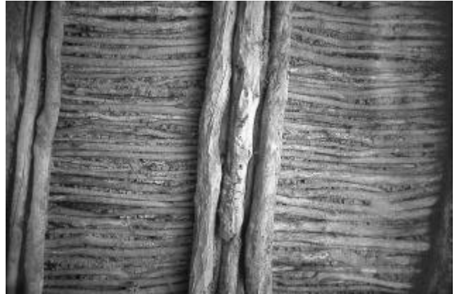
Fig. 2 Timber in a flat roof of a house in the Sahel: vast quantities of beams and branches are used.
