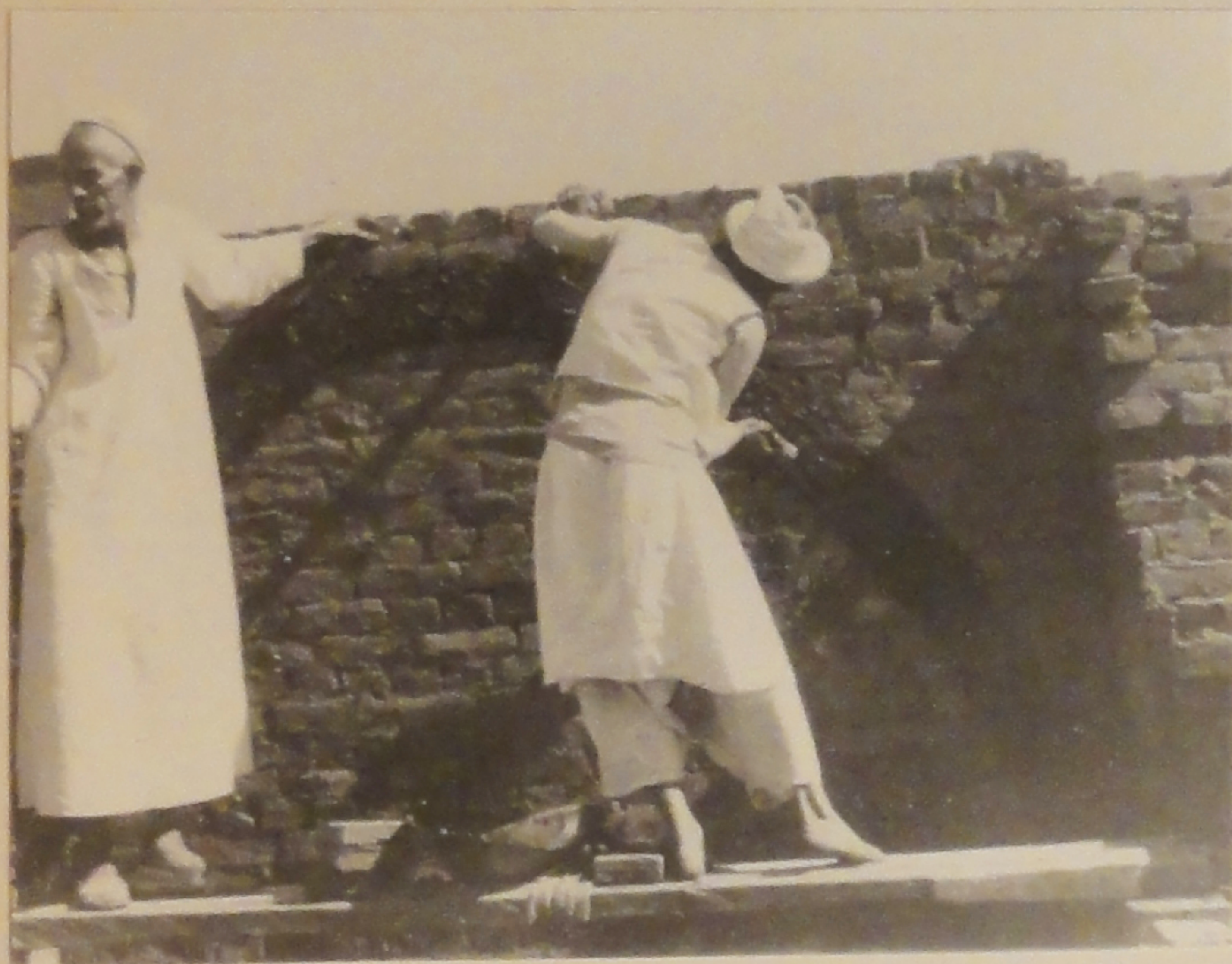
10 VAULTS ARE BUILT ON TWO SIDE WALLS AND LEANING AGAINST AN END WALL. TWO MASONS WILL WORK TOGETHER ON BUILDING IT. STANDING ON A COUPLE OF PLANKS, THEY TAKE UP HANDFULS OF MUD MORTAR (IT SHOULD BE STICKY IN TEXTURE AND OF ALMOST PURE CLAY, MIXED WITH LARGER PROPORTIONS OF STRAW WHICH WILL HAVE BEEN FERMENTING FOR TWO DAYS BEFORE BEING USED).
