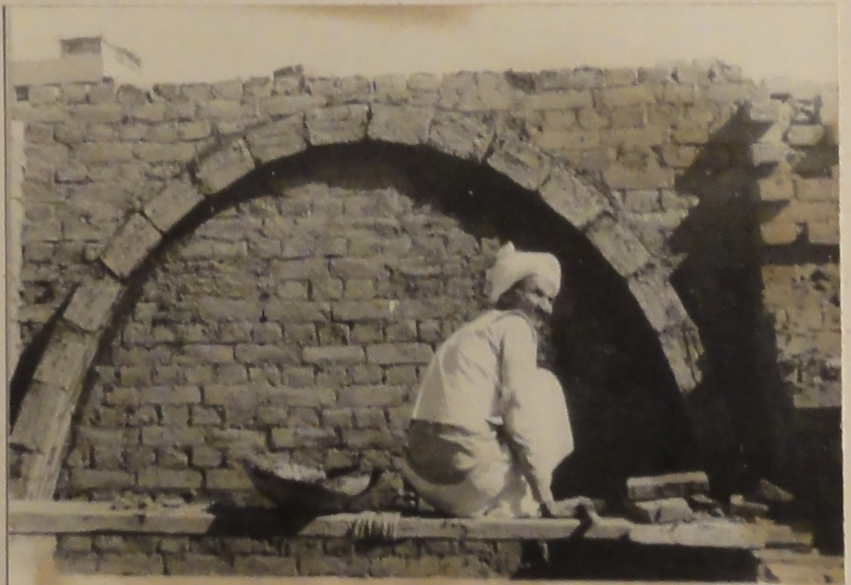
18 THE PHOTOGRAPH SHOWS THE FIRST COMPLETE PARABOLA. AT THIS STAGE THE VAULT WOULD BE SIX BRICKS THICK AT THE BOTTOM AND ONLY ONE AT THE TOP. SMALL STONES ARE TAPPED INTO THE GAPS BETWEEN THE BRICKS TO ENSURE THAN THE VAULT IS UNDER COMPRESSION.
