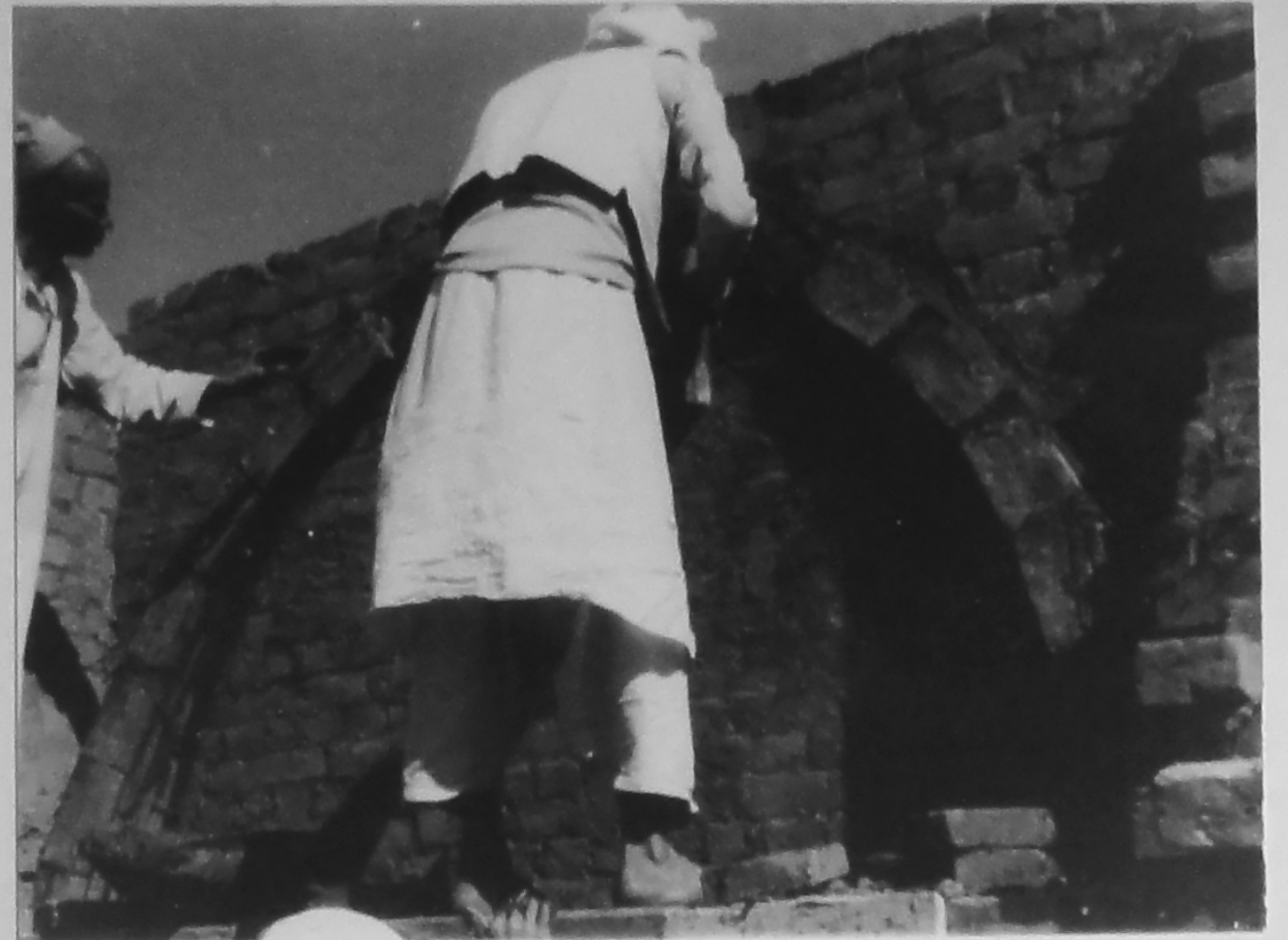
16 & 17 THESE TWO PHOTOGRAPHS SHOW THE TWO MASONS GRADUALLY BUILDING THE INCLINED COURSES OUT, EACH ONE RISING A LITTLE HIGHER ROUND THE OUTLINE OF THE PARABOLA, TILL THE TWO CURVED LINES OF BRICK MEET AT THE TOP.
