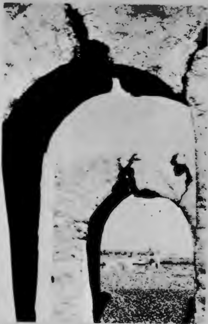
Sabra-cracked arches on first floor
