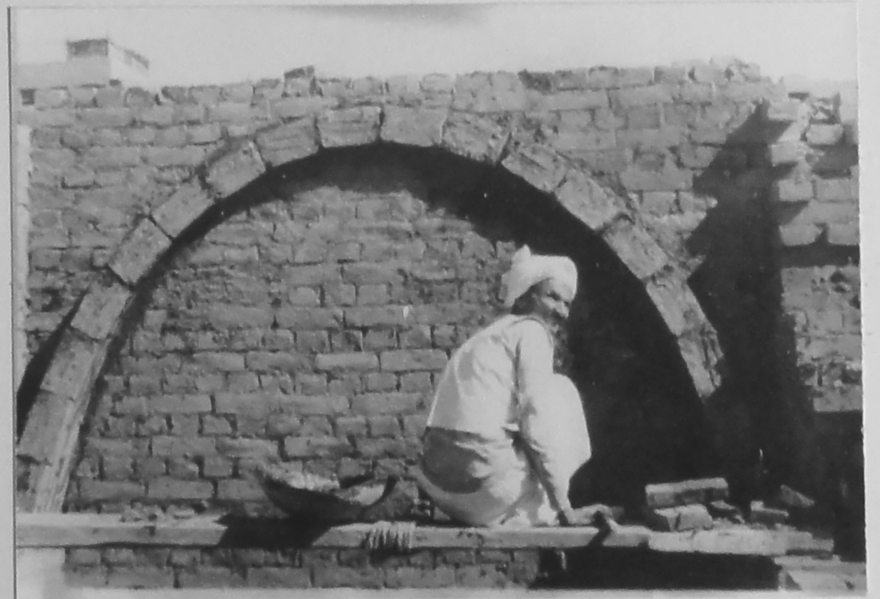
18 THE PHOTOGRAPH SHOWS THE FIRST COMPLETE PARABOLA. AT THIS STAGE THE VAULT WOULD BE SIX BRICKS THICK AT THE BOTTOM AND ONLY ONE AT THE TOP. SMALL STONES ARE TAPPED INTO THE GAPS BETWEEN THE BRICKS TO ENSURE THAN THE VAULT IS UNDER COMPRESSION.
