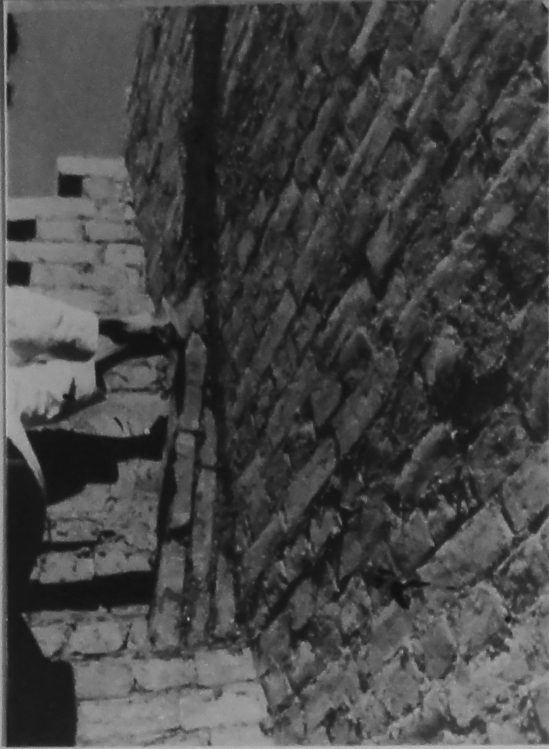
14 THE MASONS NOW PUT IN MORE MUD PACKING AGAINST THE SECOND COURSE, SO THAT THE THIRD COURSE WILL INCLINE EVEN MORE ACCUTELY THAN THE SECOND. THE THIRD COURSE IS THREE BRICKS HIGH.
