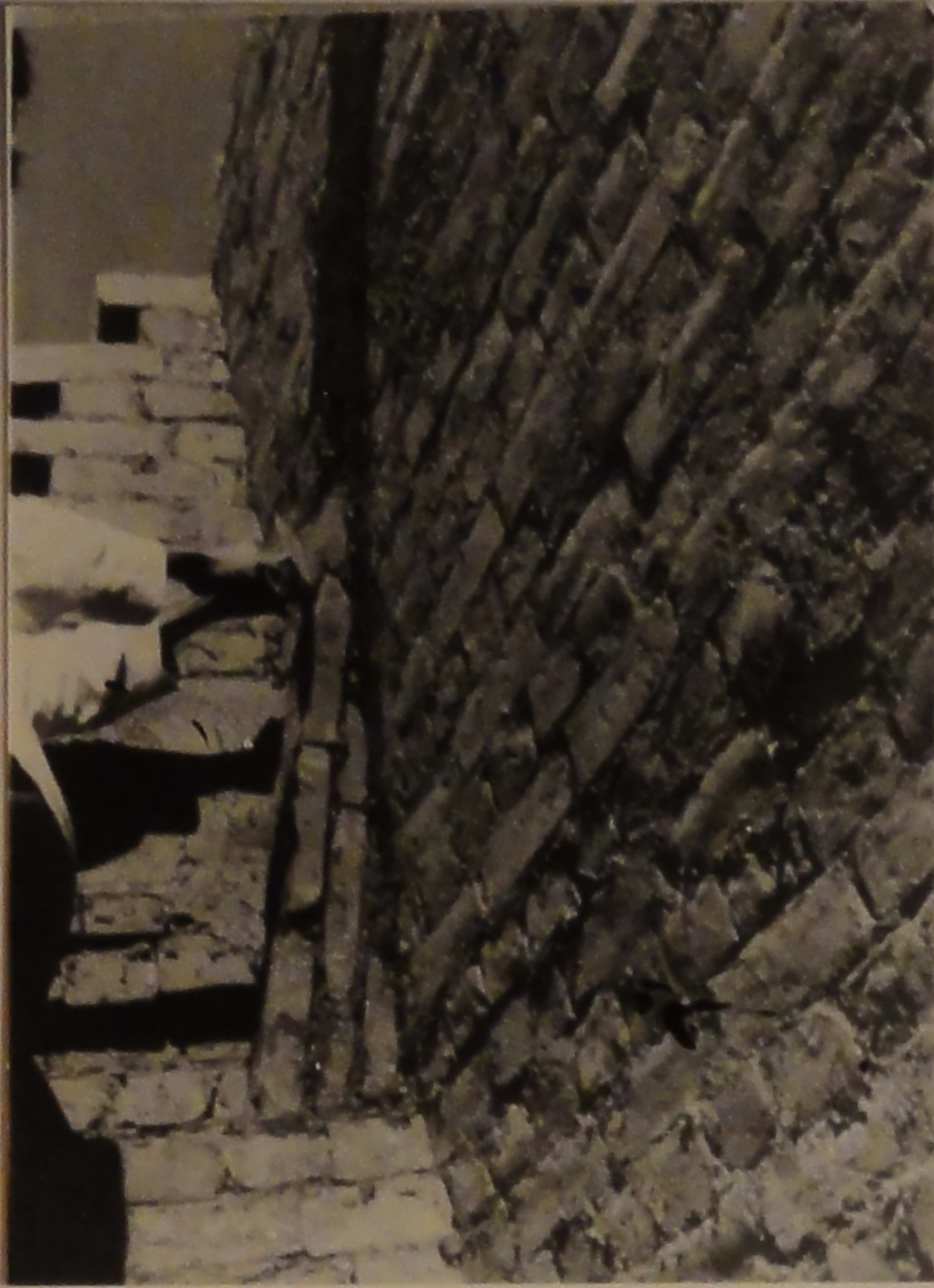
14 THE MASONS NOW PUT IN MORE MUD PACKING AGAINST THE SECOND COURSE, SO THAT THE THIRD COURSE WILL INCLINE EVEN MORE ACCUTELY THAN THE SECOND. THE THIRD COURSE IS THREE BRICKS HIGH.
