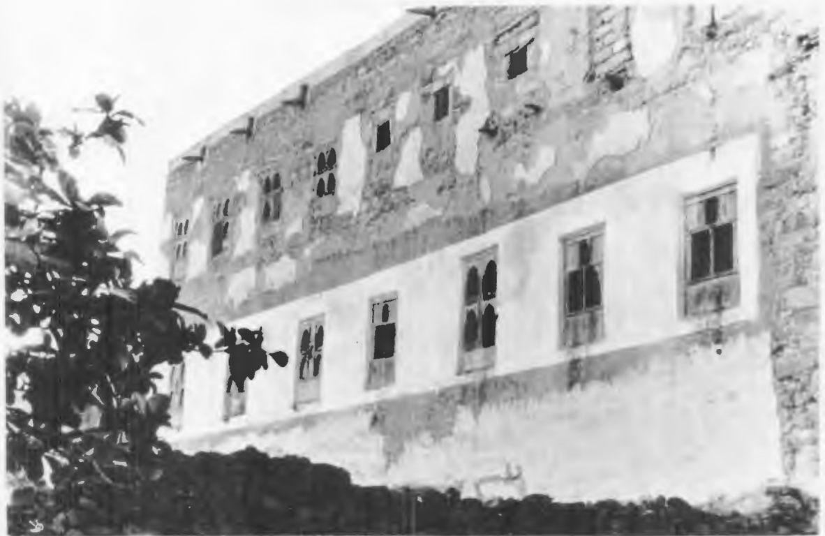
One of the oldest town houses in Salala (18 th century), though in disrepair.
