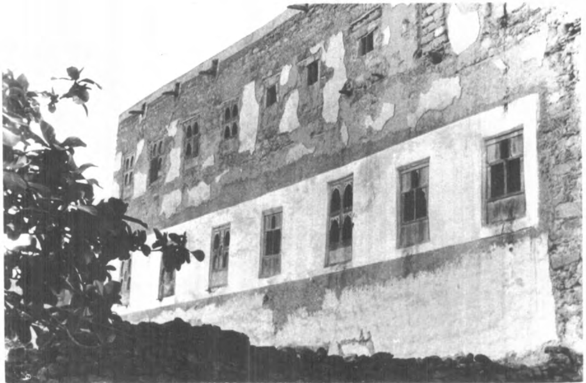
One of the oldest town houses in Salala (18 th century), though in disrepair.
